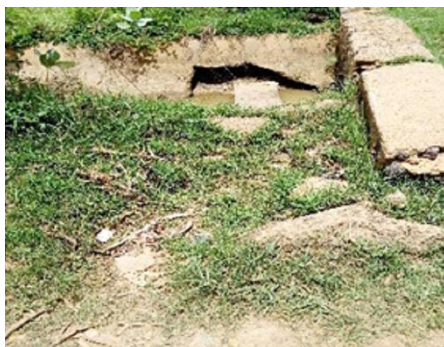
Figure 4: Degradation of irrigation canals
