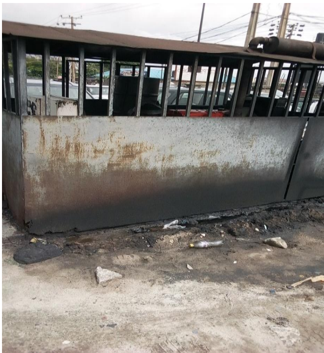
Plate 1: Private Electricity Generator in Front a shop.
