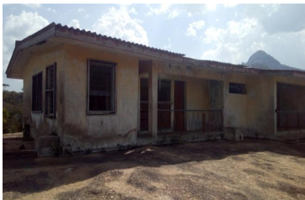
Figure 3: Guest/Tourist Chalet in poor condition, Oke Idanre.
