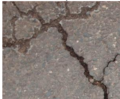
Figure: 1 Cracks healed with calcium carbonate Source: Society for Applied Microbiology
